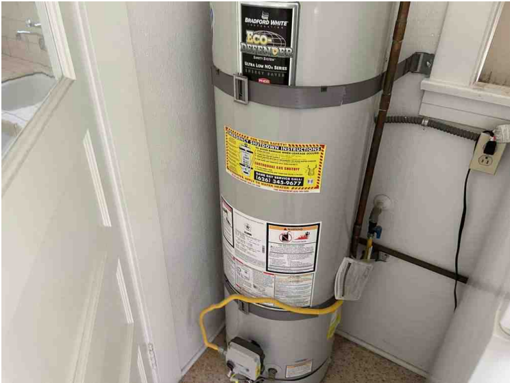
Hot Water Heater Unit "A"
