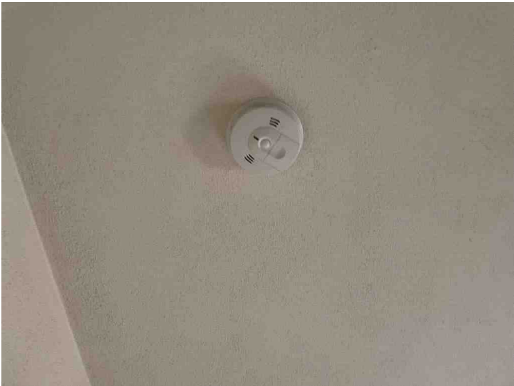
Smoke & Carbon Monoxide Detector Combo Unit "C"
