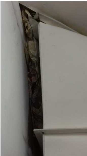
Existing Library ducting sealed with newspaper from the 1980's
