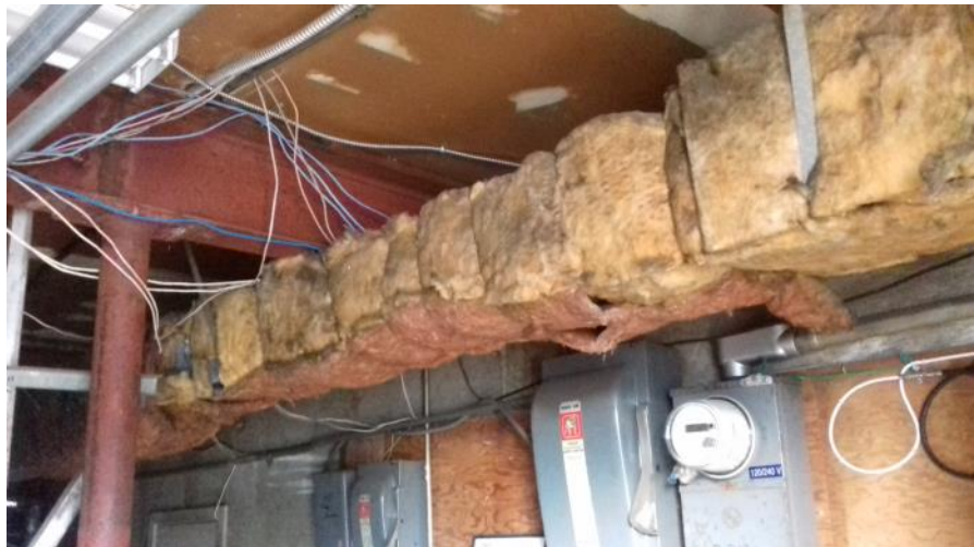
Deferred ductwork and antiquated electrical work underneath the Library.
