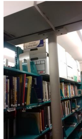
Support beams set awkwardly amidst storage shelving in the Library basement.
