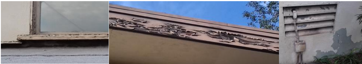
Peeling paint, eroded window fittings, cracks in stucco, and evidence of dry rot are all indications of repairs that are long overdue.
