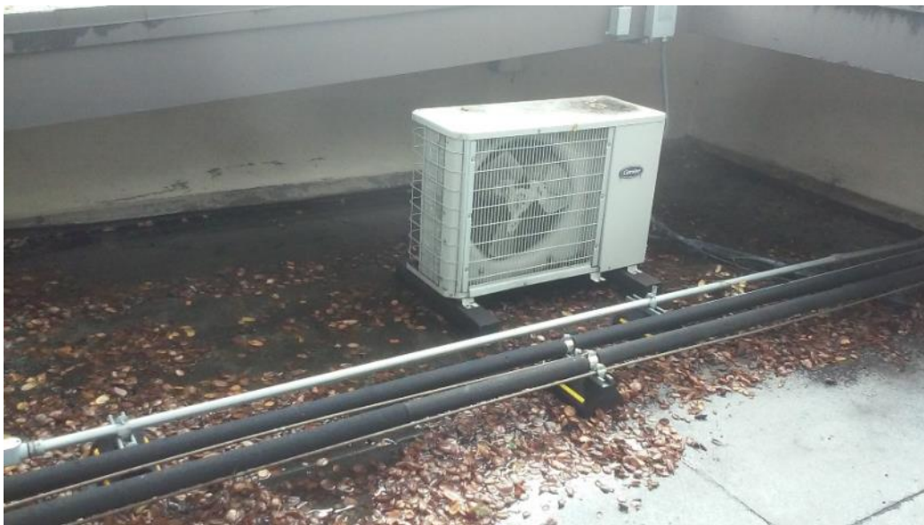
Water collects on a negatively sloped area of the Library roof that does not have drainage. At 3 inches deep, the water must be hand swept off of the roof after rain.
